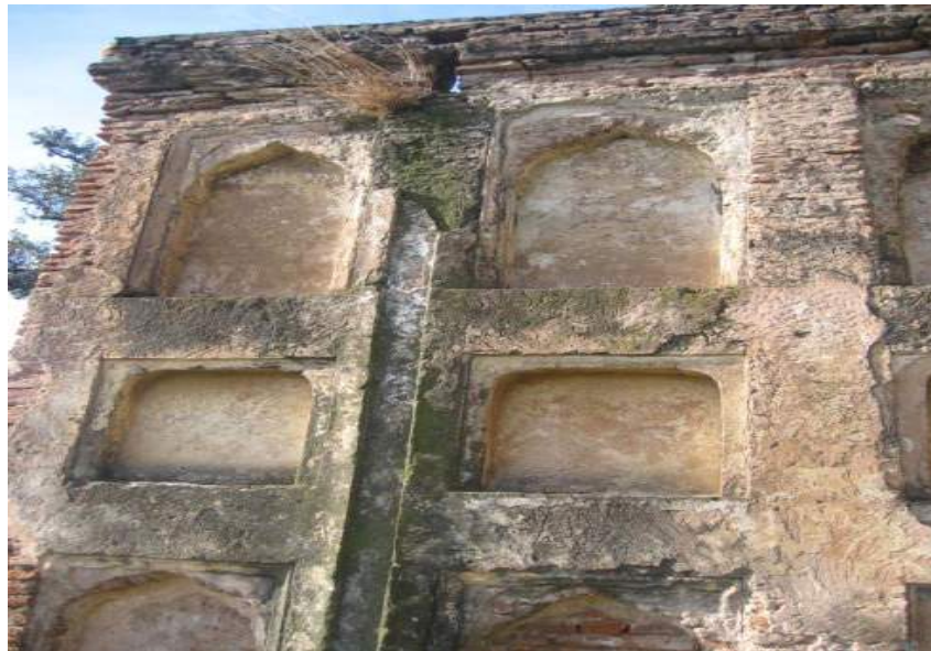
Pl. II: Guli Bagh: Broken water shut the improper flow of rainwater and growth of fungus
