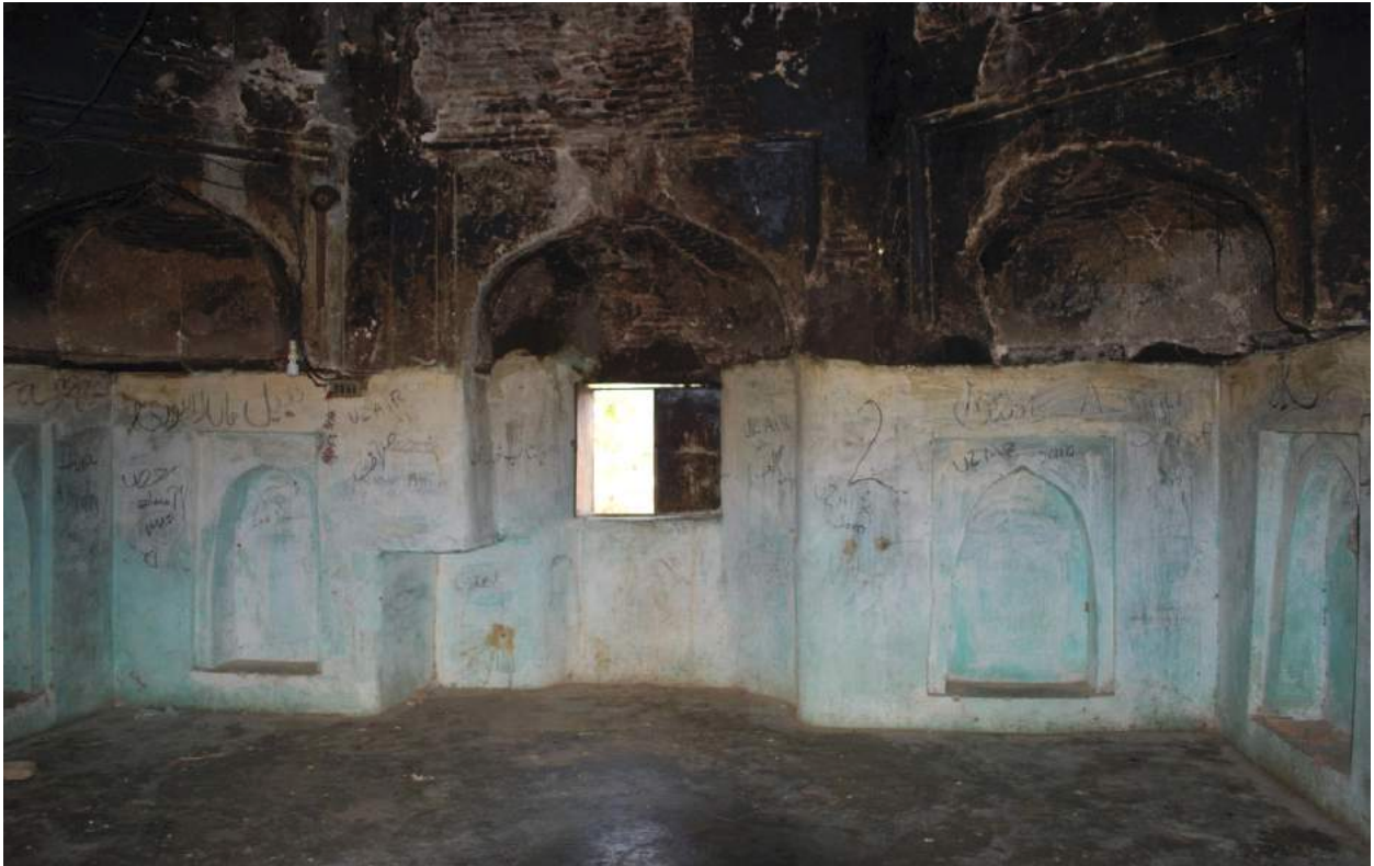
Pl. V: Guli Bagh: Detail of interior removed plaster badly damaged due to ravages of time
