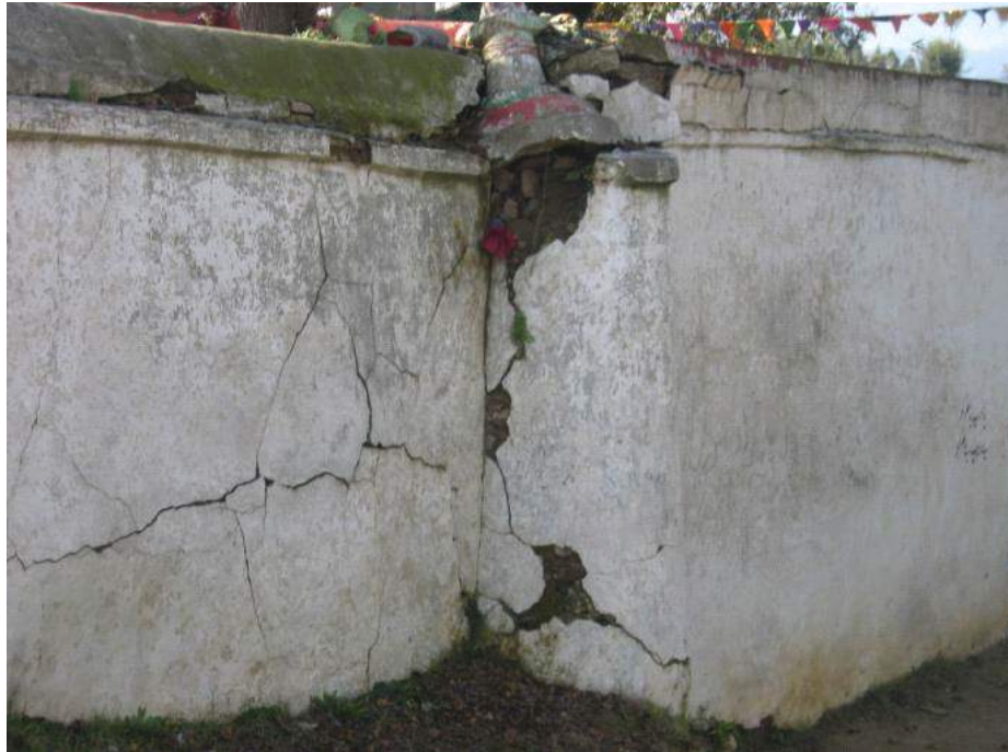
Pl. III: Guli Bagh: Close up of Northern bastion showing cracks and missing parts
